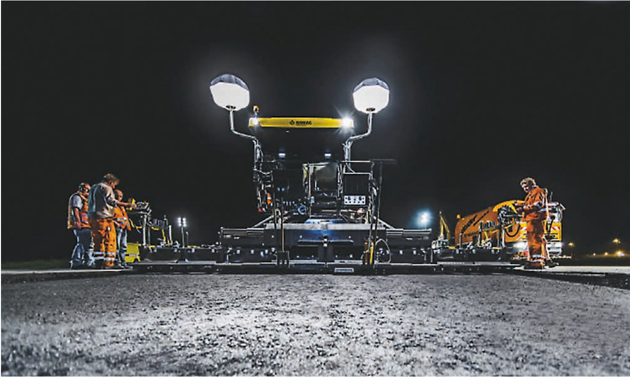
Perfect evenness as a result—especially when under time constraints such as here on a night time construction site at the airport.
