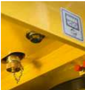
Highly visible markings on service points
