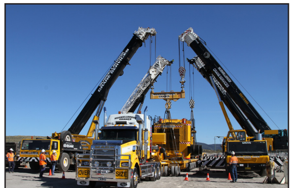
Above - Utilising an equalising beam, the 2 x 160 tonne, 1 x 140 tonne & 1 x 100 tonne slew cranes unloaded the main frame upon arrival at Bulga Mine
