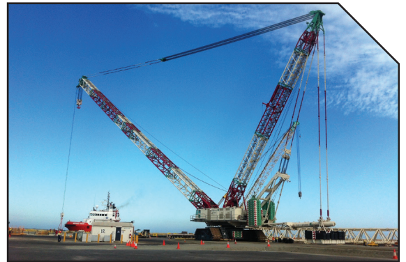
Above - The Terex-Demag CC8800-1 setup and readied for the major moves and lifts.
