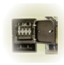
Connection Termination Box
