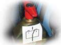
Battery Isolating Switch
