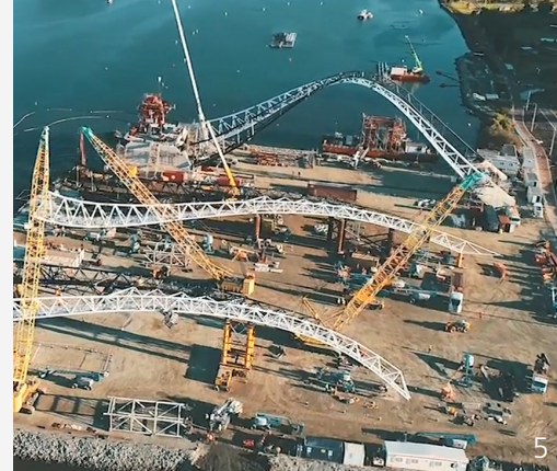
Images - 1. Load-out and assembly of the Deck Modules. 2. Two SCX2800-2, 275t Hitachi Sumitomo Crawlers Cranes, carrying out dual crane operation for the load-out of Arch sections for Span 2. 3. MLC650 VPC MAX, 700t Manitowoc Crawler Crane with variable positioning counterweights, lifting a 140t deck module for load-out. 4 & 5. Construction and assembly of the arch spans. 6. (following page) MLC650 VPC MAX (700T Crawler Crane), SCX2000A-2 (200T Crawler Crane), 2 x SCX2800-2 (275t Crawler cranes).
