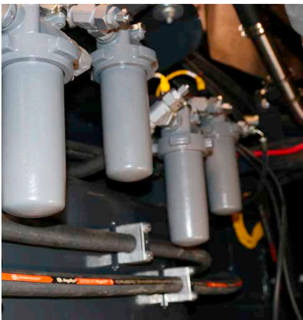
Hydraulic filter system.
