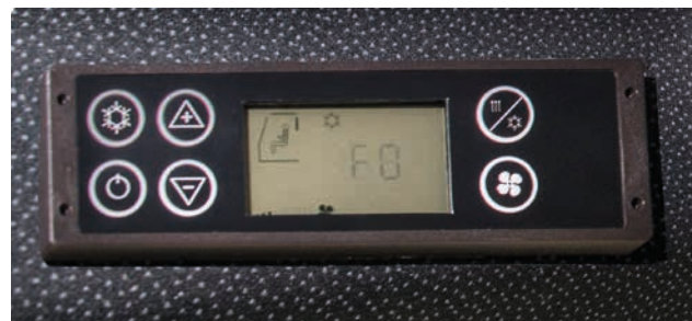
Automatic heating and air-conditioning unit control panel.
