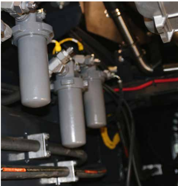
Hydraulic filter system.
